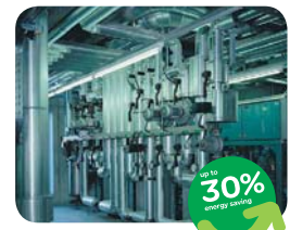
Application of ATV12 in a pumping station
